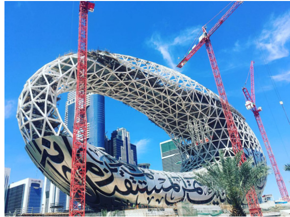
Figure 2: The construction site of the Museum of Future in Dubai. The photo was taken by the author on March 20th, 2019..
